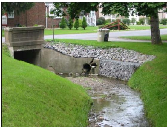
Streambank stabilization project on Tub Mill Run required as a result of excessive stormwater runoff
